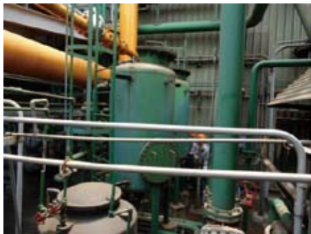
“A major iron manufacturing company” (Large sand filter X 2)
