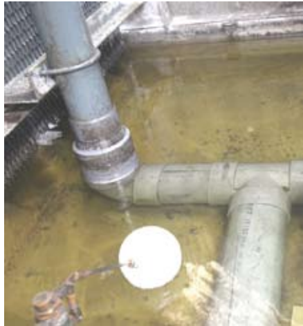
Inside cooling tower with CALFA"SEP"
