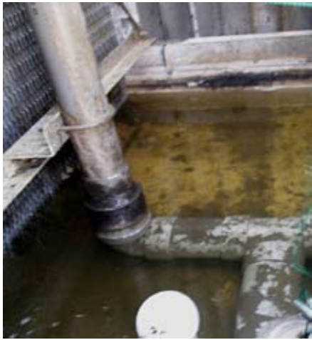
Inside cooling tower without CALFA"SEP"
